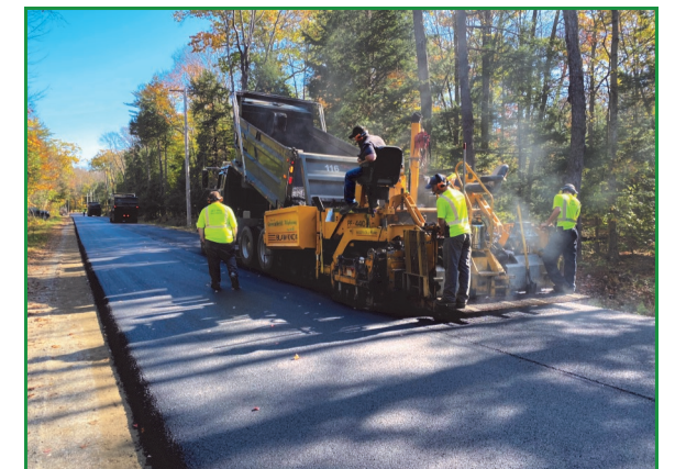
Our highway team at work. Summer hours for the Town Highway Department are 6 a.m.-4:30 p.m. Monday—Thursday.
